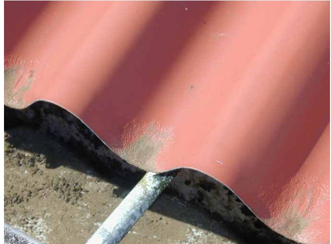
Silt accumulation on a panel without a drip edge. Blistering of the paint is an early sign of corrosion.
