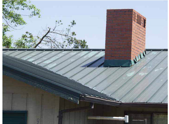
Excessive use of touch-up paint that has faded faster than factory applied coating.
