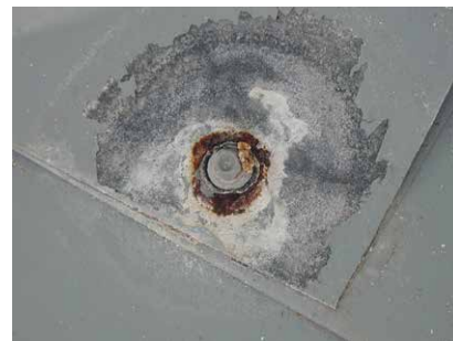
Over driven fastener resulting in premature corrosion of the ZINCALUME panel.
