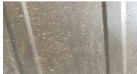
Heavy swarf staining on pre-painted ZINCALUME.
