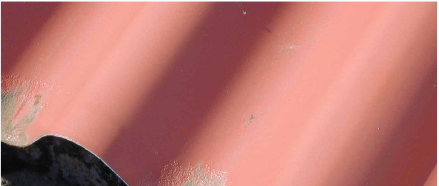
Silt accumulation on a panel without a drip edge. Blistering of the paint is an early sign of corrosion.
