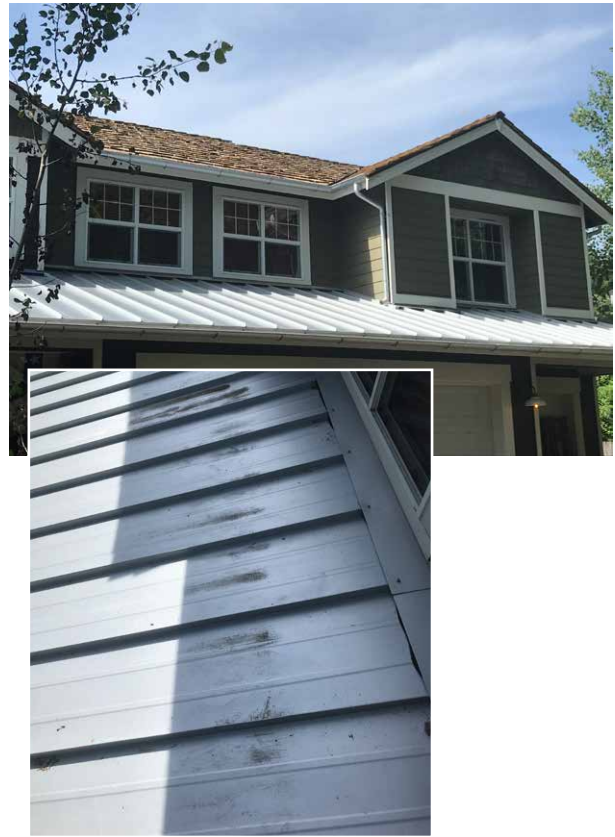
Copper treated shingles above bare ZINCALUME roof panels, the water runoff resulted in black oxidation.
